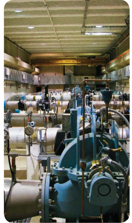
Eramosa designed and programmed the automated control system for this water pumping station capable of pumping over 900L/s of potable water for one of Ontario’s largest municipalities.
